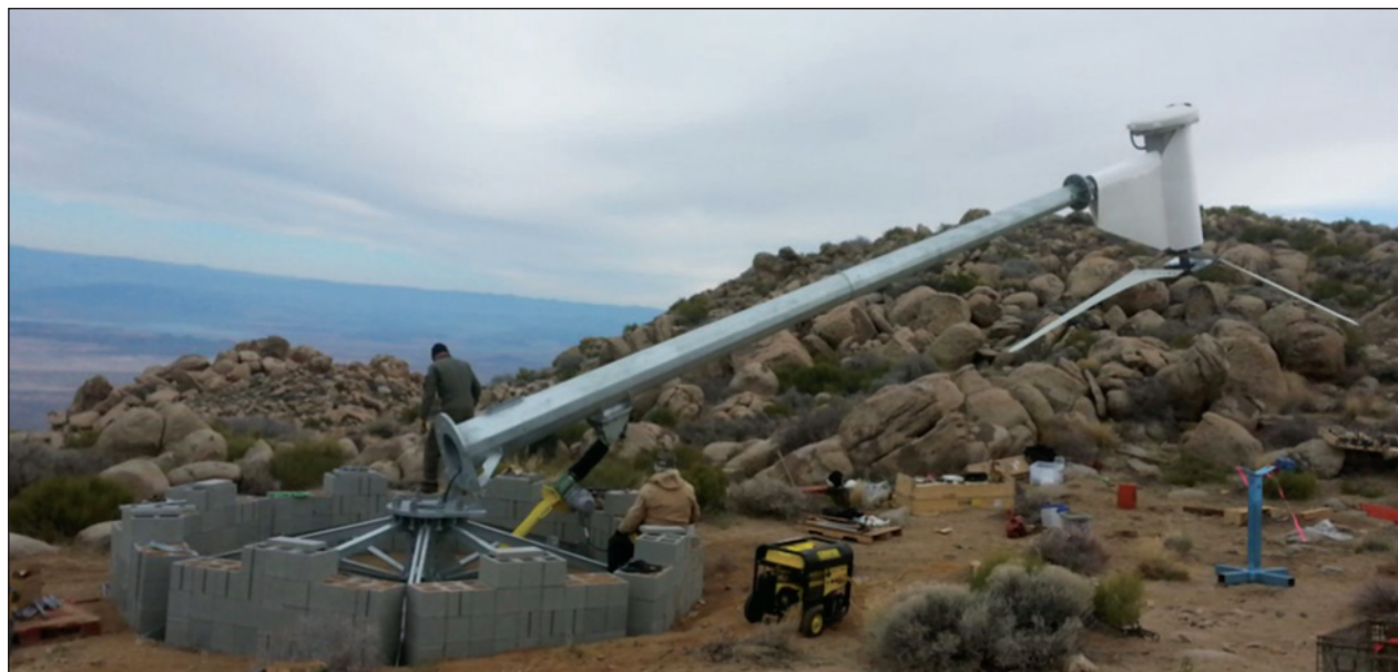
Figure 6. Installation of SD wind turbine on a rock surface (SD Wind Energy Limited, 2019)
