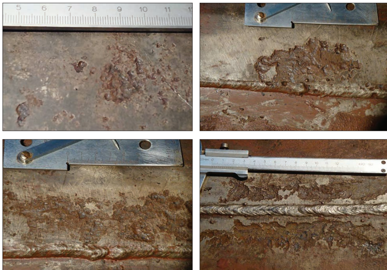
Figure 3. General view of corrosion damage at the tank's bottom
